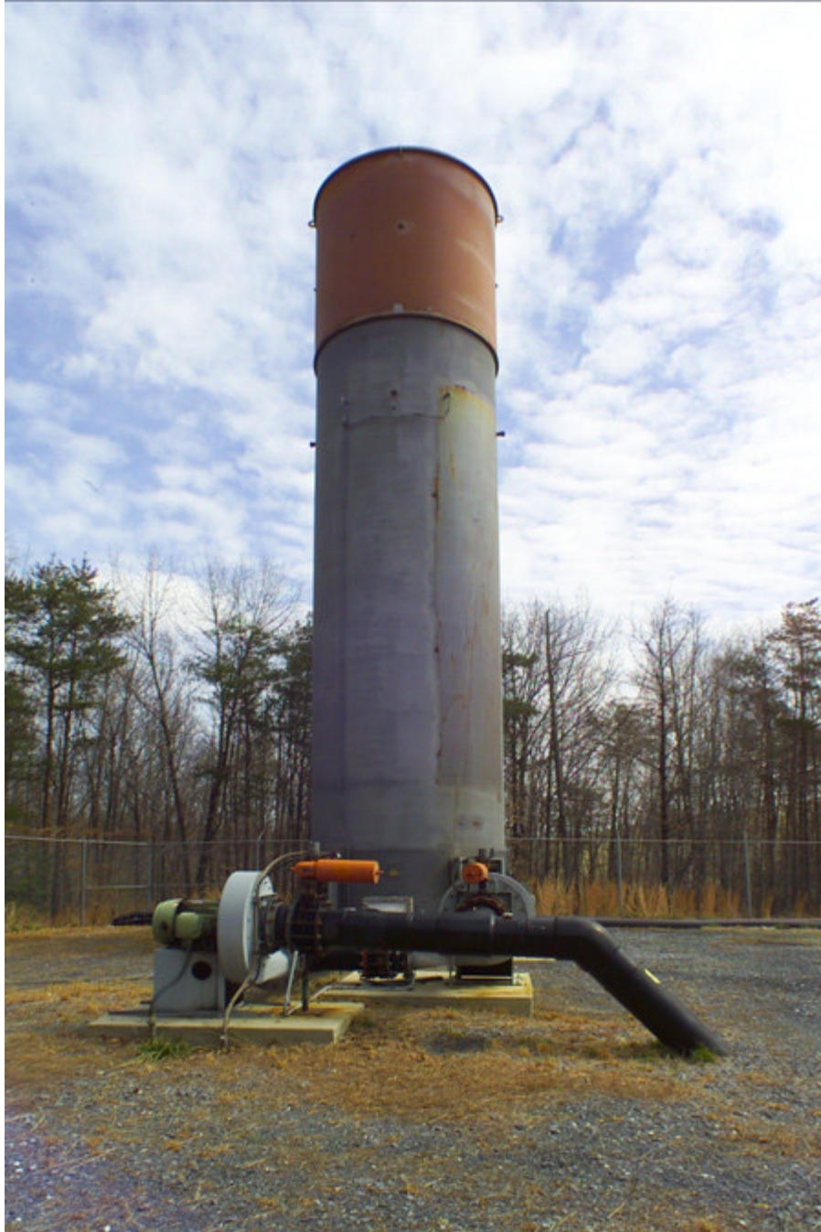
Typical Landfill Gas Flare 2
